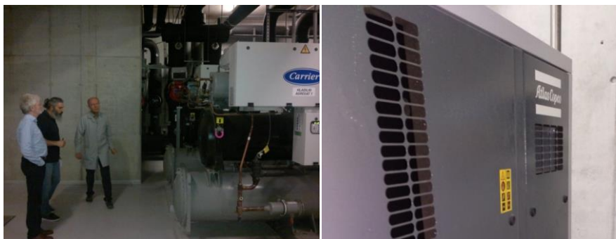
Figure 11: Technical room in the basement (left) and Air treatment detail (right).
