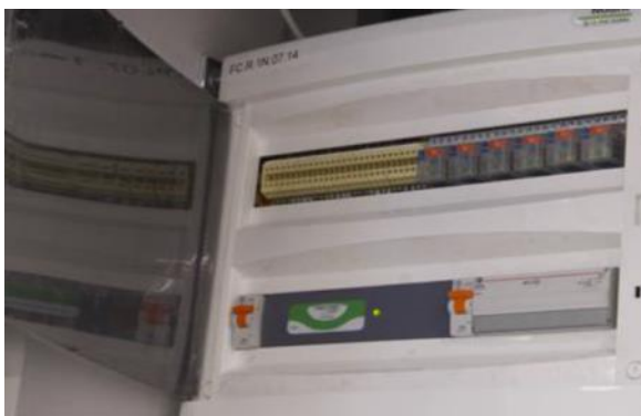
Figure 6: Image of room automation PLC.
