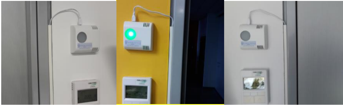
Figure 5: Existing thermostats (Honeywell CentralLine) already present in all the rooms for UL.
